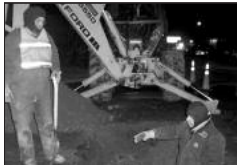
Water servicer Ed Glasberg (left) and Distribution Manager John Speciale (right) in a trench preparing to fix a water main break.
